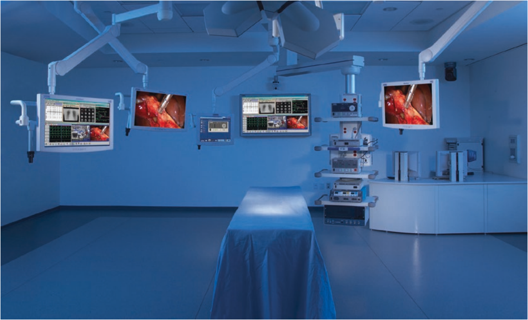
Fig. 2.1 Integrated operating room ORI™, KARL STORZ
